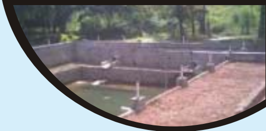
RWH reservoir at 8th Bn. Machenahalli, Shimoga Dist.
